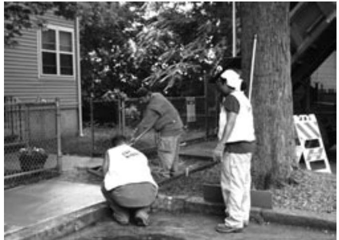
DPW sidewalk crews repair a concrete sidewalk on Harrington Terrace. In-house crews completed close to 300 such repairs last year.
