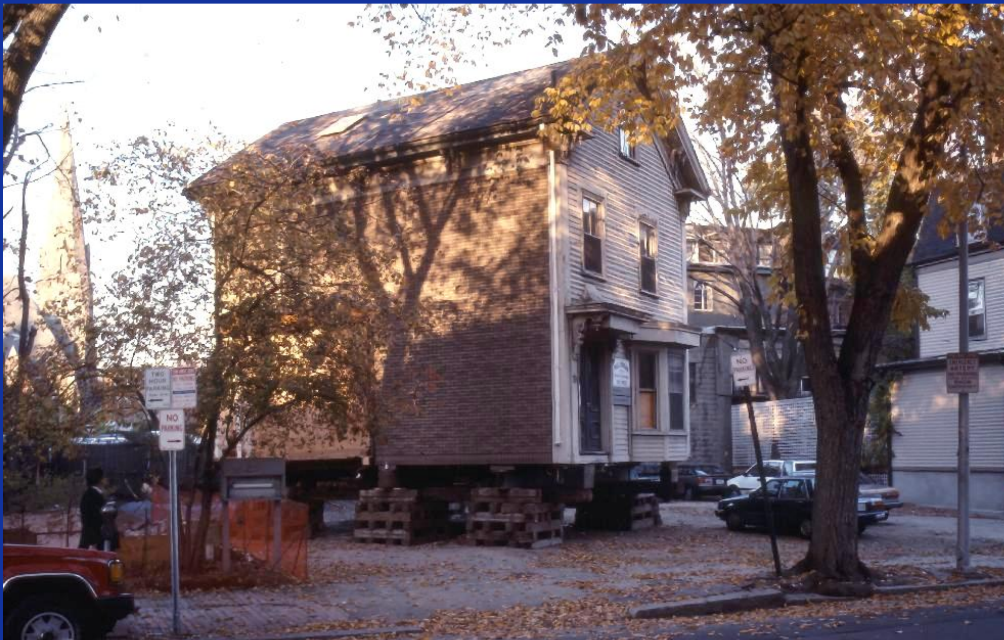
19 Mt. Auburn Street, October 26, 1988
