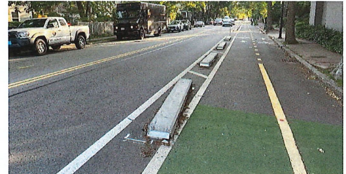
A precast curb was dislodged near Fresh Pond Parkway where there was a missing delineator post. (2025)
