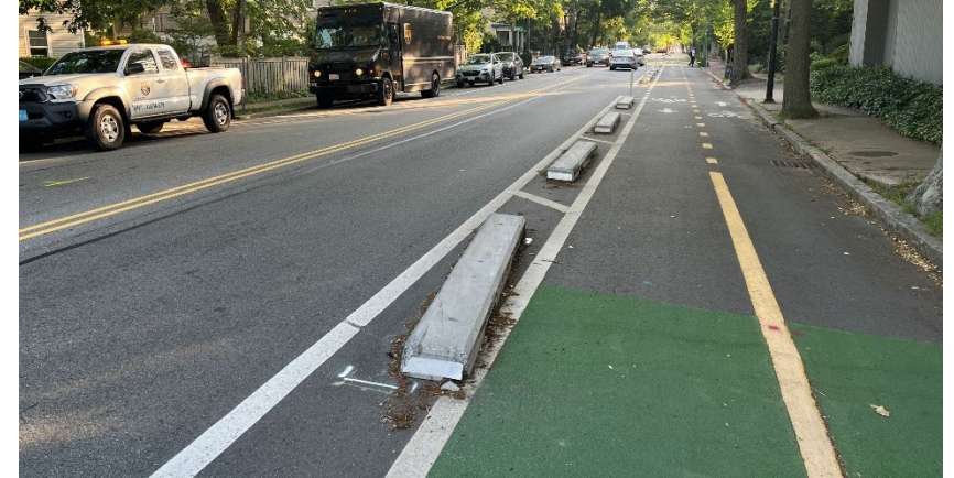
A precast curb was dislodged near Fresh Pond Parkway where there was a missing delineator post. (2025)
