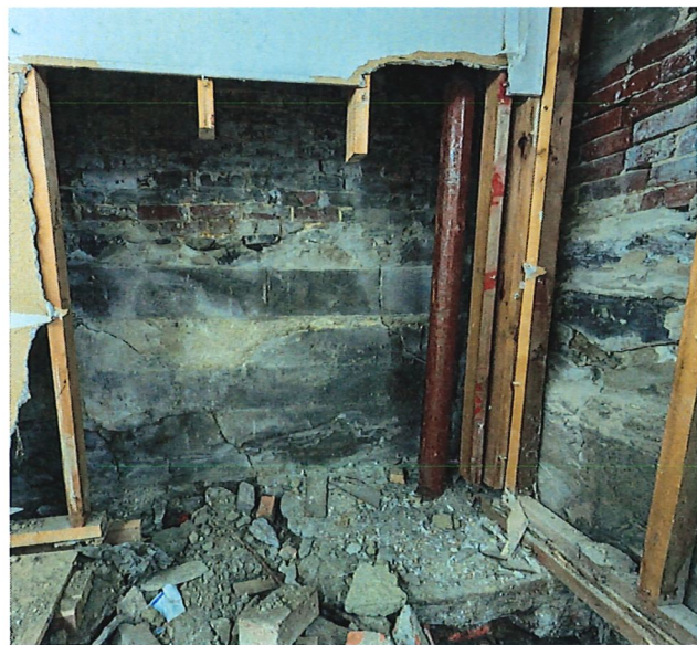
COMPROMISED FOUNDATION WALL
