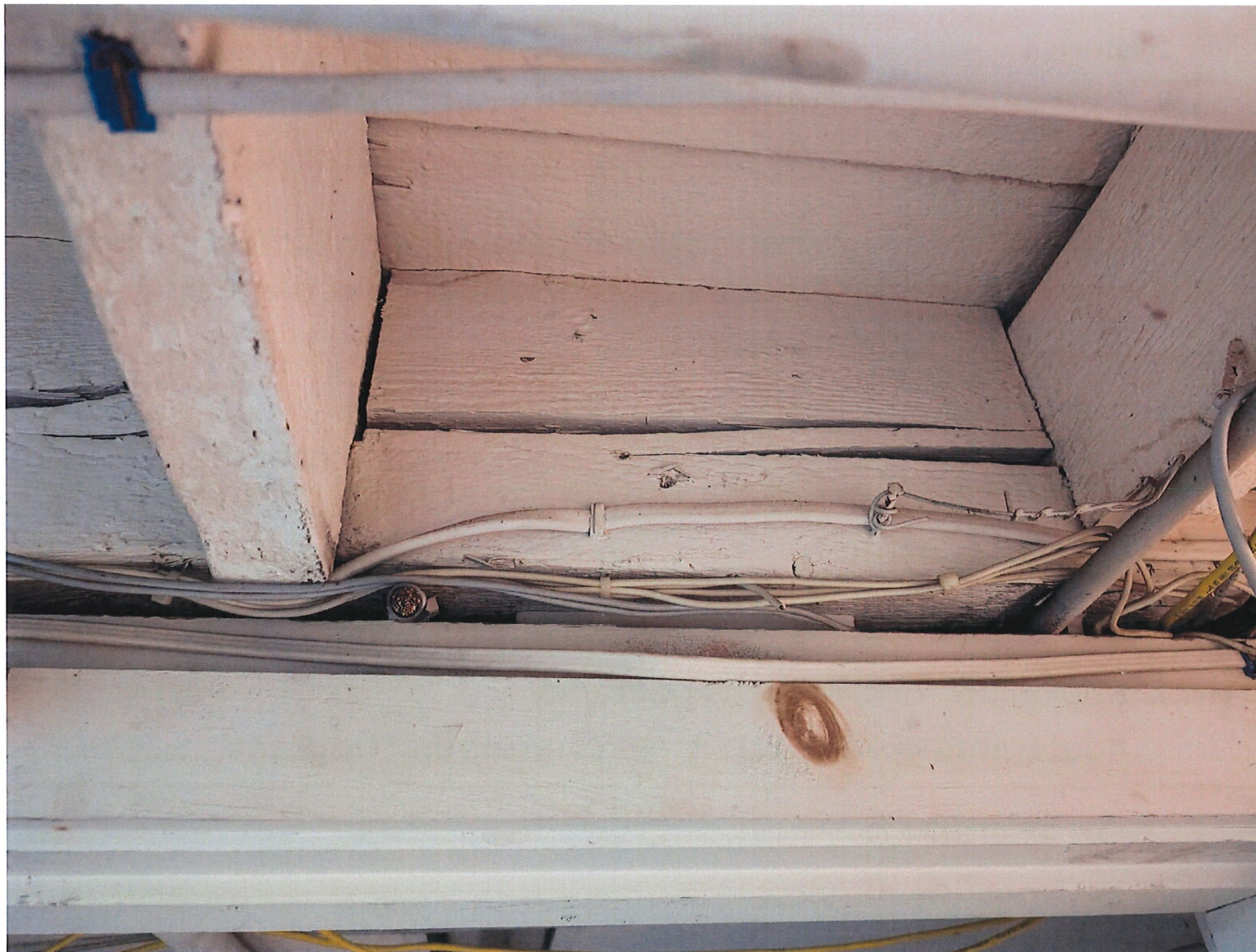
COMPROMISED FLOOR FRAMING BEAM
