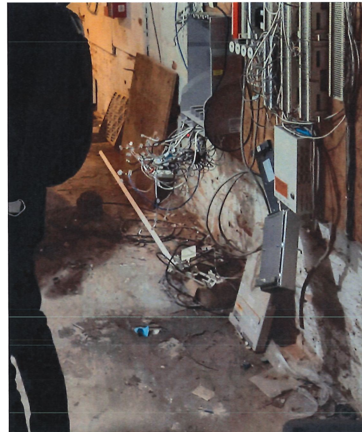
WATER INFILTRATION AT SLAB
