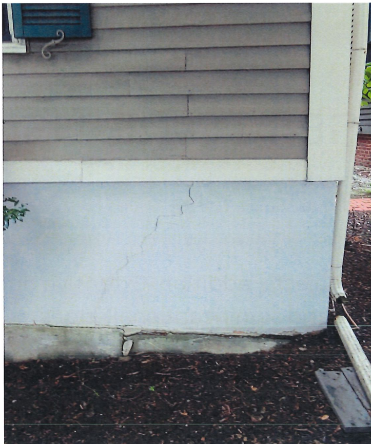
EXISTING FOUNDATION CRACKS/ BILLOWING
