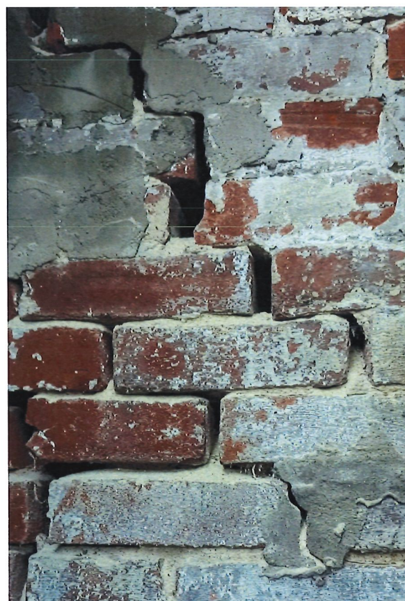
DETERIORATED MASONRY AT FOUNDATION WALL
