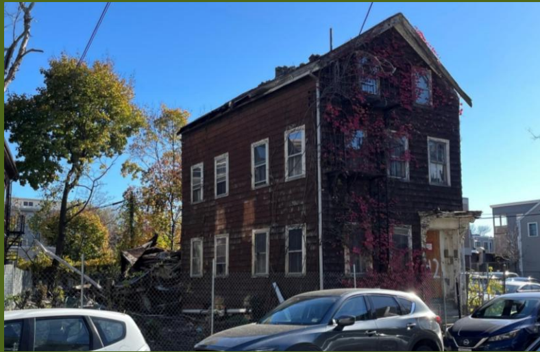
Partially collapsed building
