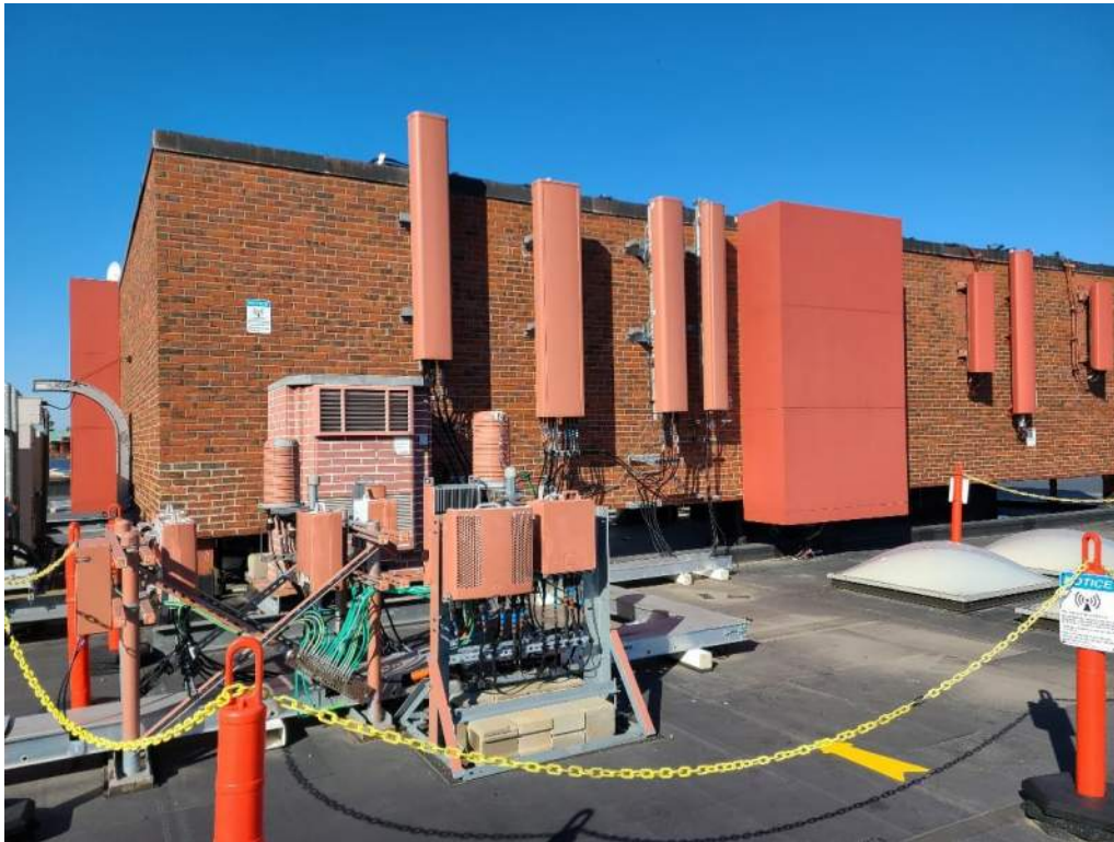
Photo 1: Sample photo illustrating the existing Alpha & Beta sector antennas.
