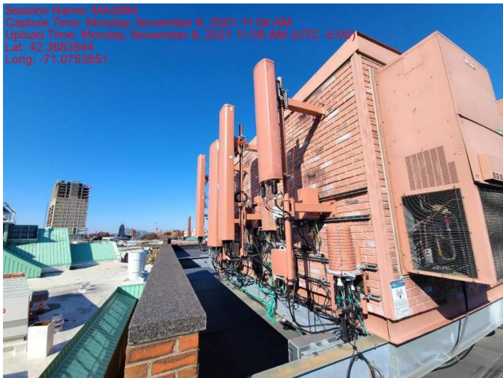
Photo 2: Sample photo illustrating the existing Gamma sector antennas.
