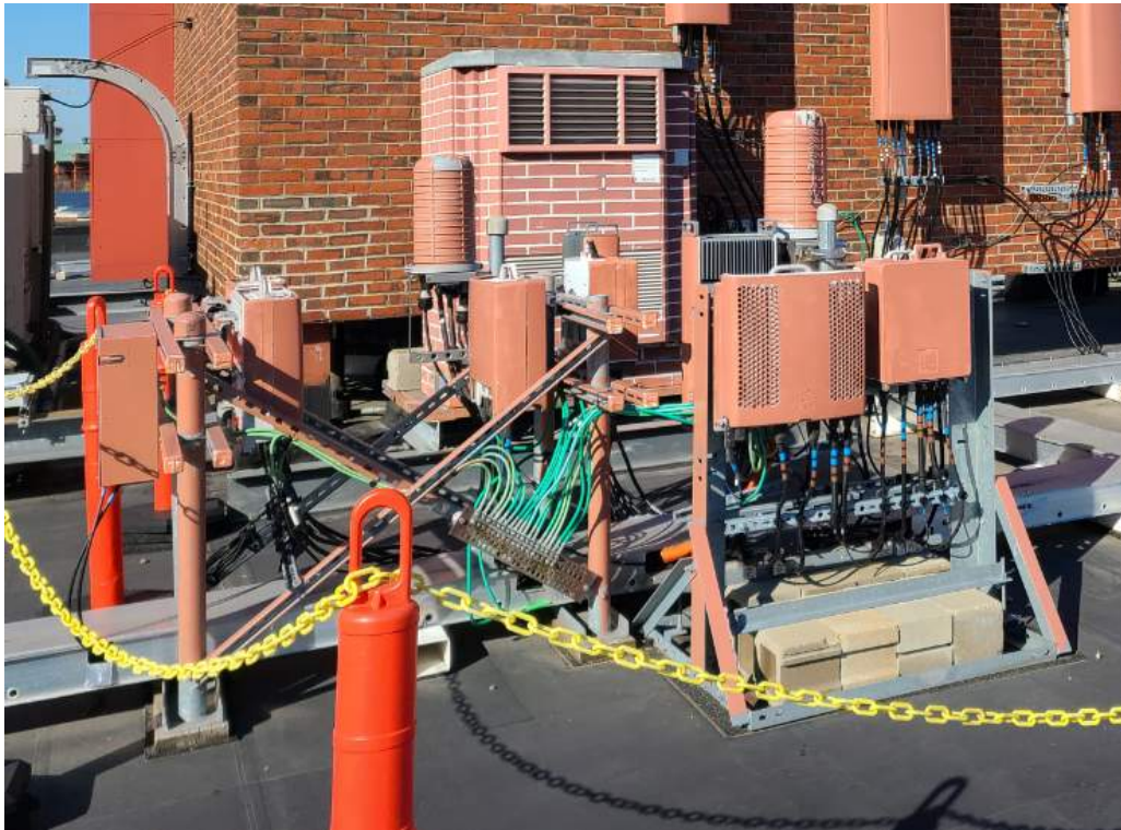
Photo 3: Sample photo illustrating the existing RRH ballast sleds.
