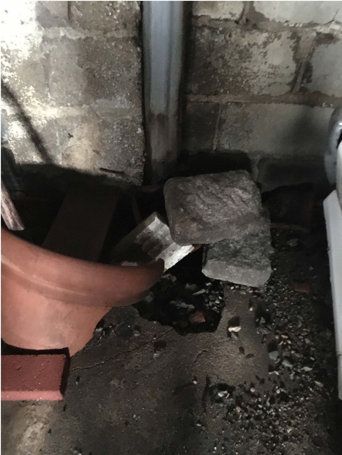
Cracking at slab-on-grade foundation
