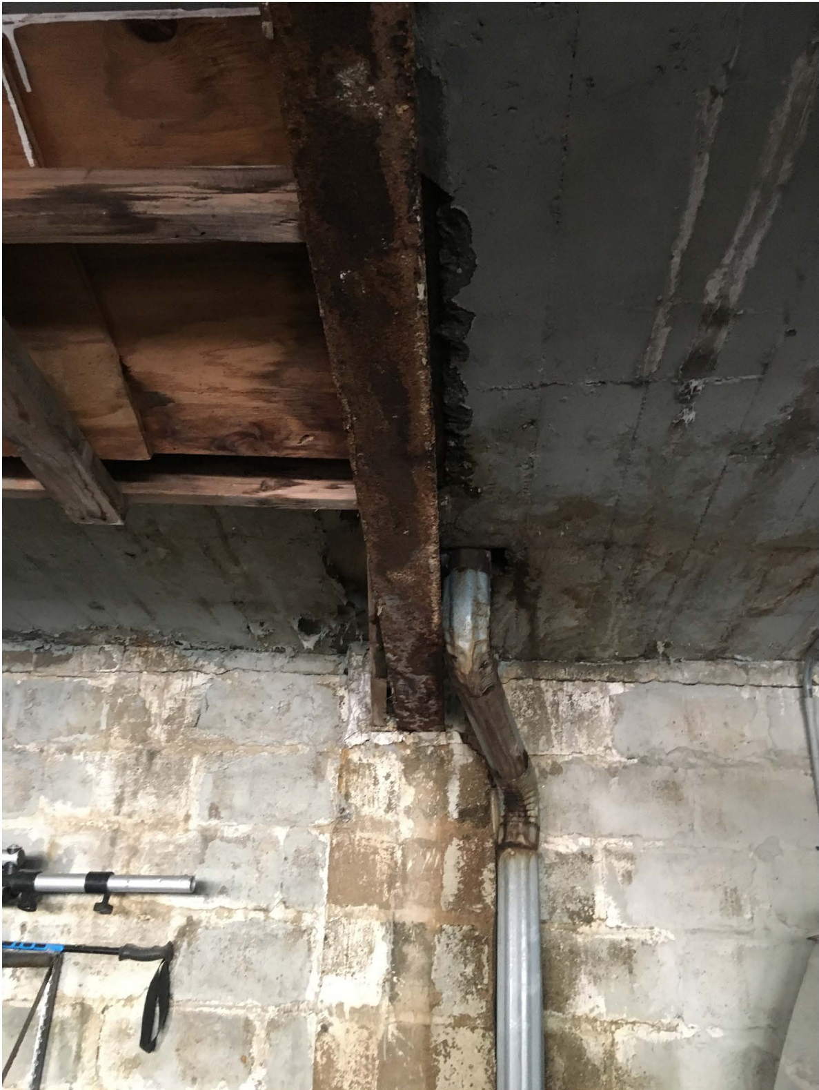
Deterioration at structural steel beam
