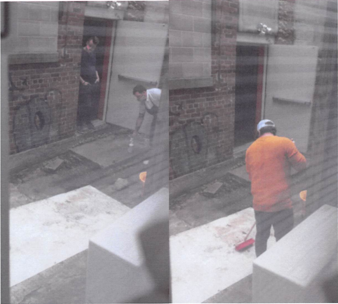
May 9, 2020: use of the rear alley to clean plastic floor mat with chemicals
