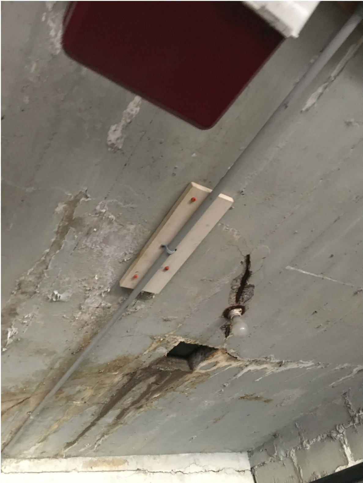
Concrete rot at ceiling with oxidized exposed rebar
