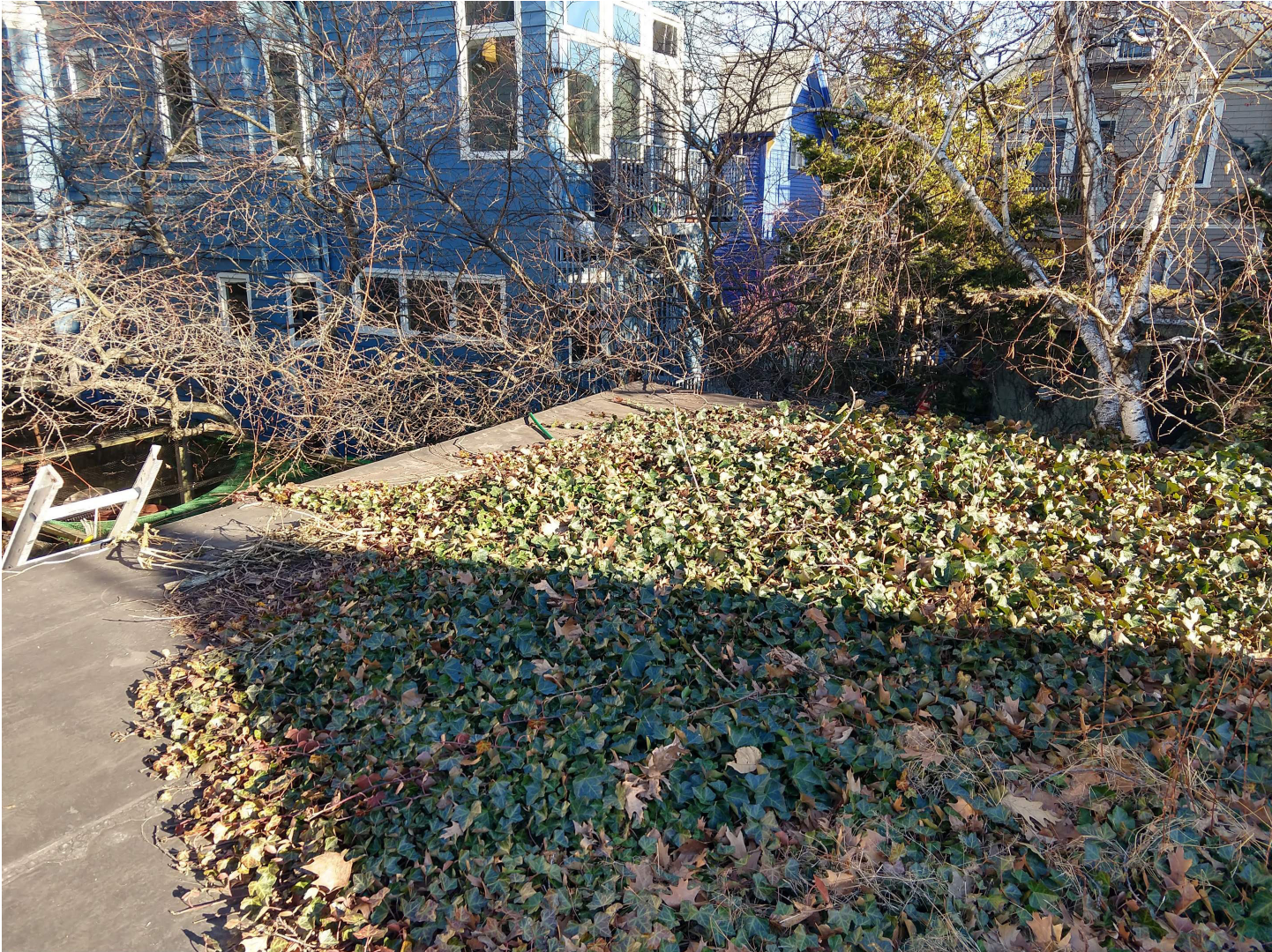
Ivy and moss degrading EPDM roof membrane. Green roof is proposed in this area.
