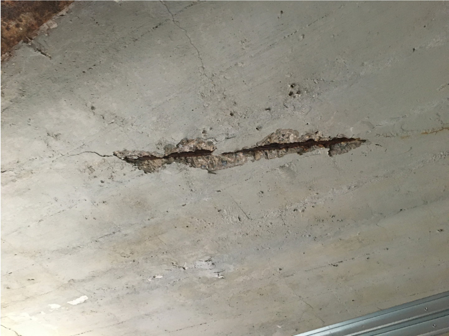
Concrete rot at ceiling with oxidized exposed rebar
