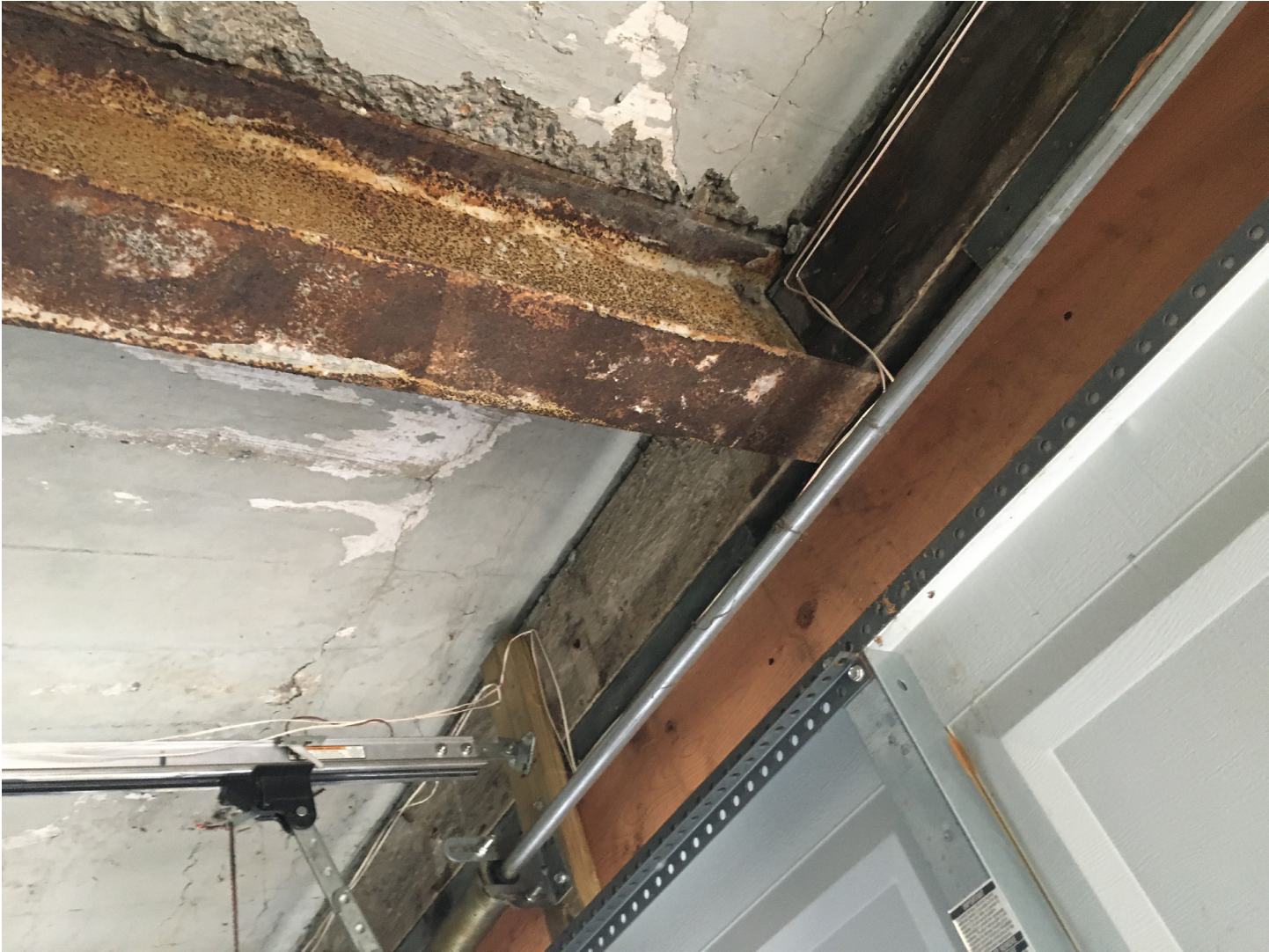
Deterioration at structural steel beam
