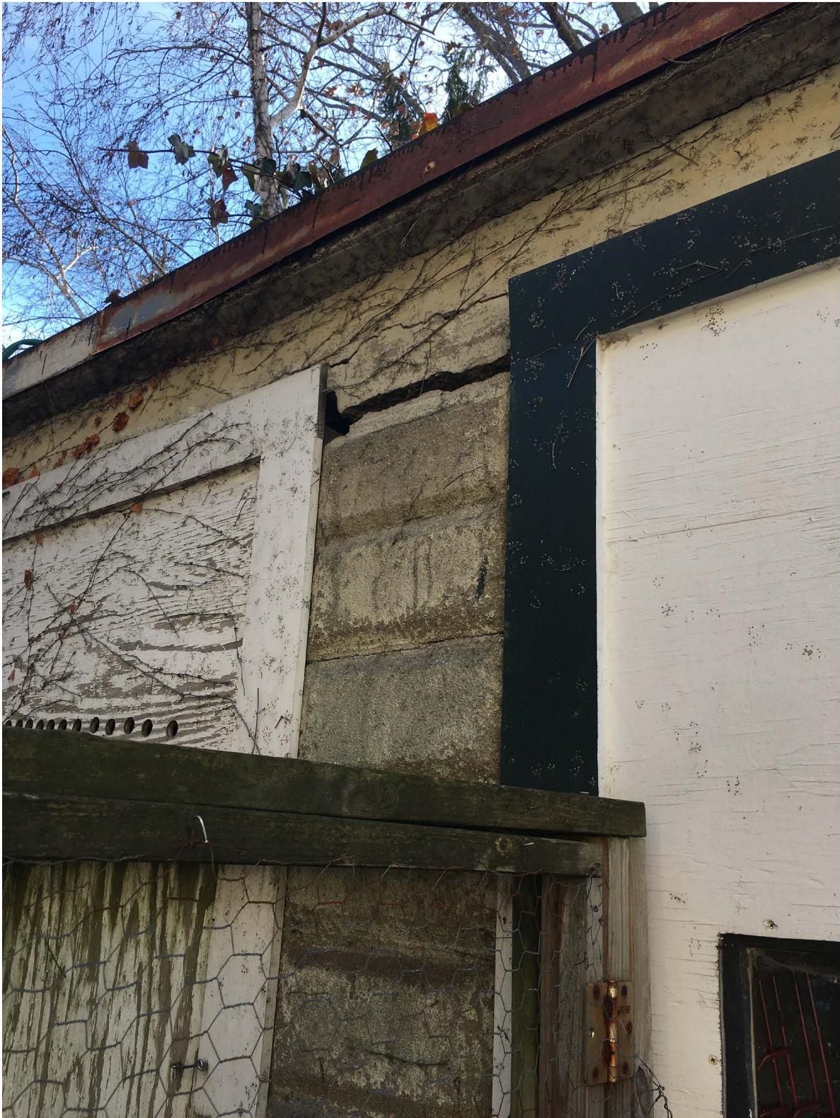
Cracking in concrete block wall
