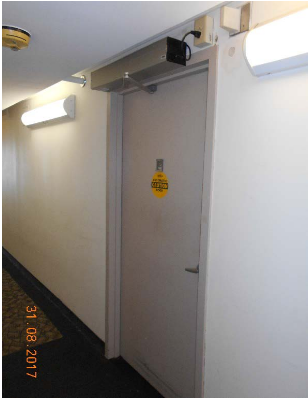
Interior Conditions 7 Typical HP Apartment Entry Door with Opener
