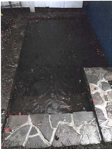
Ponding of water in stairwell to shed since construction of condos
