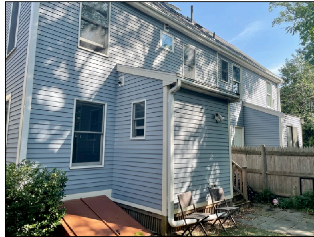
Back View from Southwest Corner (Bump out to remain and bulkhead to be removed)
