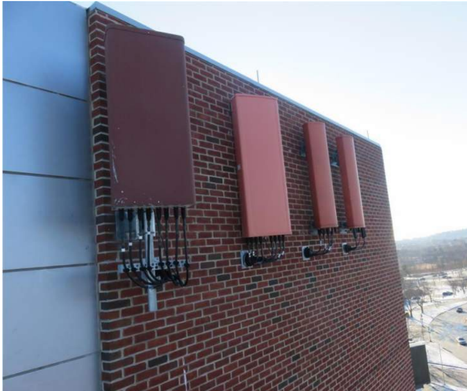
Photo 3: Sample photo illustrating the existing Gamma sector antennas.
