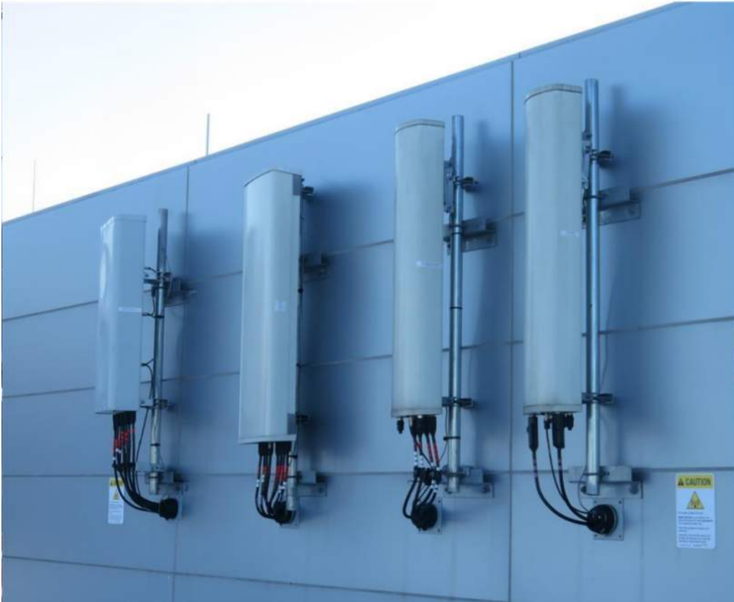
Photo 1: Sample photo illustrating the existing Alpha sector antennas.
