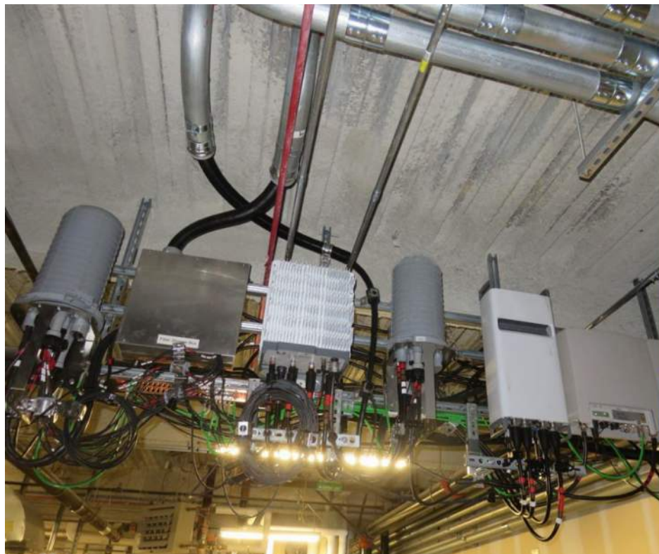
Photo 4: Sample photo illustrating the existing RRH's and surge arrestors.
