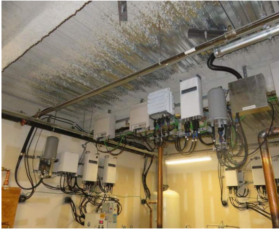
Photo 5: Sample photo illustrating the existing RRH's and surge arrestors.
