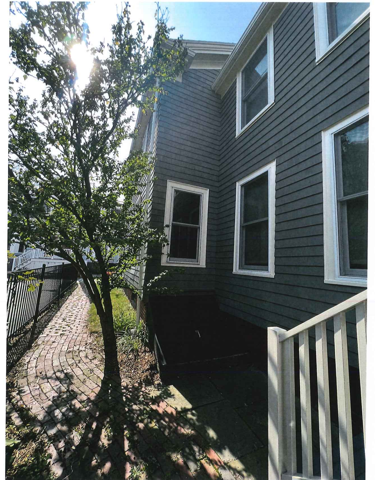
3 AMORY PLACE VIEW OF REAR FACING BULKHEAD TO BE REPLACED BY 1-STORY ADDITION
