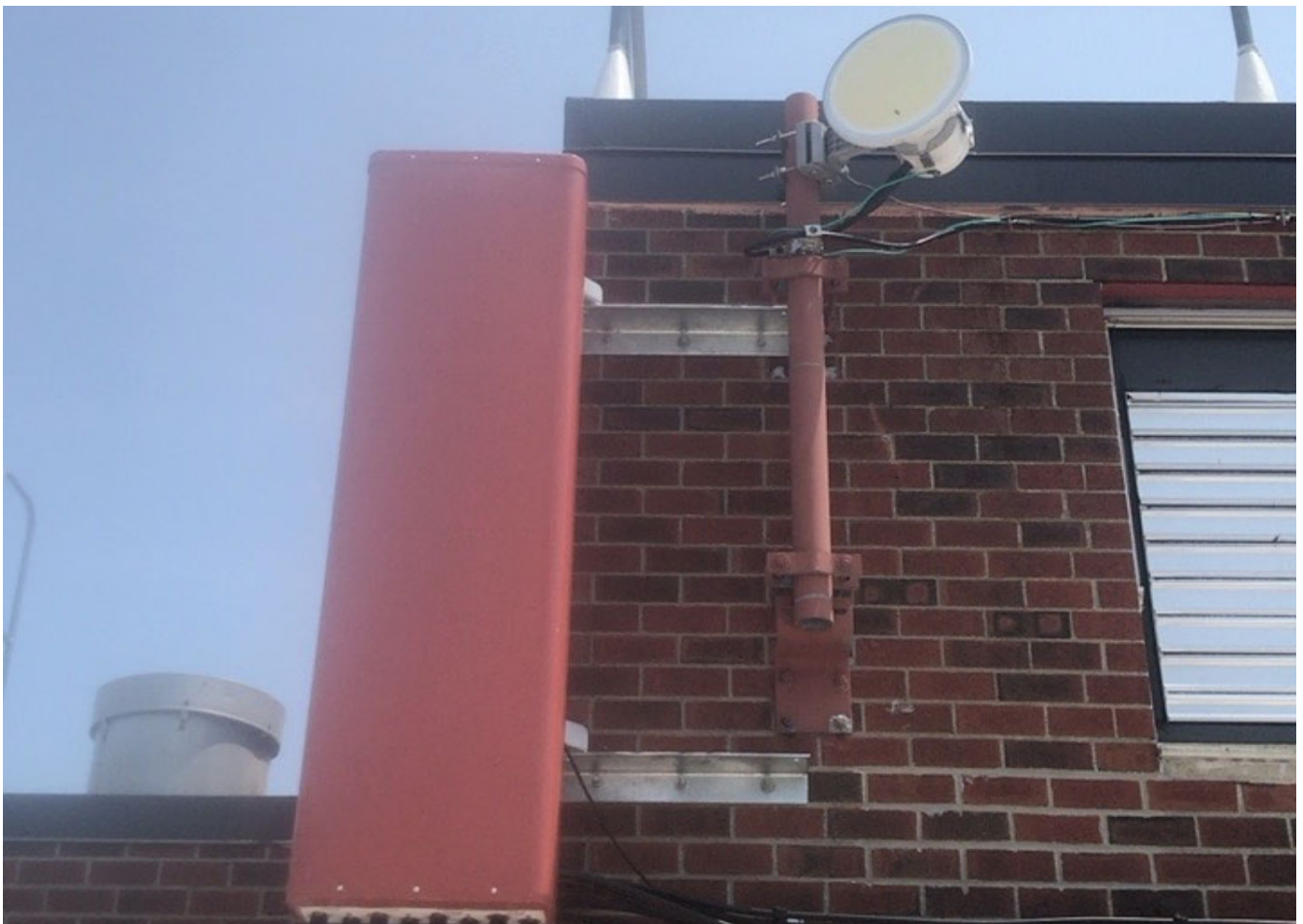
Existing Gamma Sector Antennas
