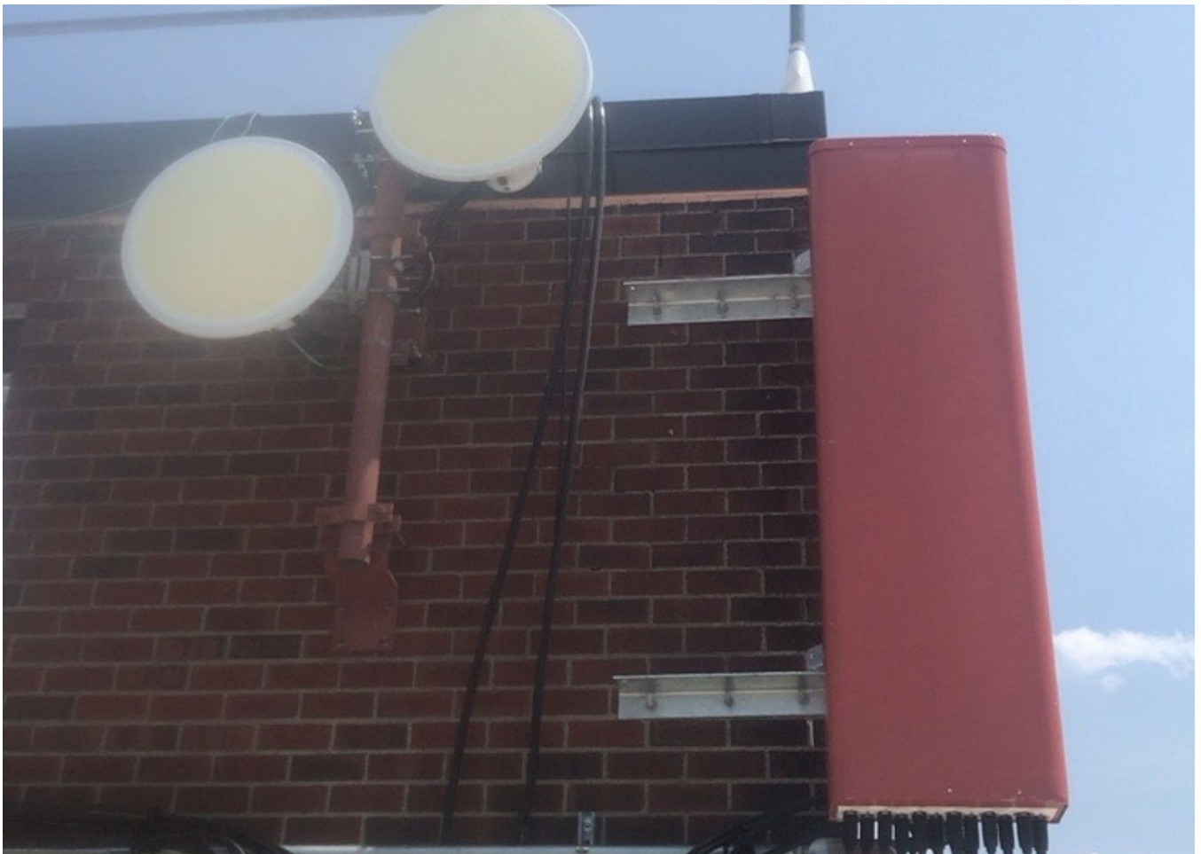
Existing Gamma Sector Antennas
