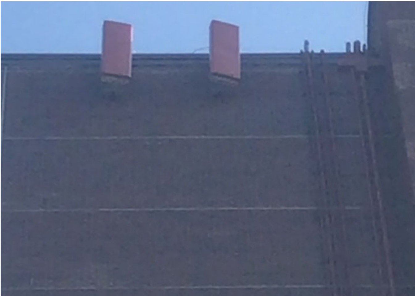
Existing Alpha Sector Antennas
