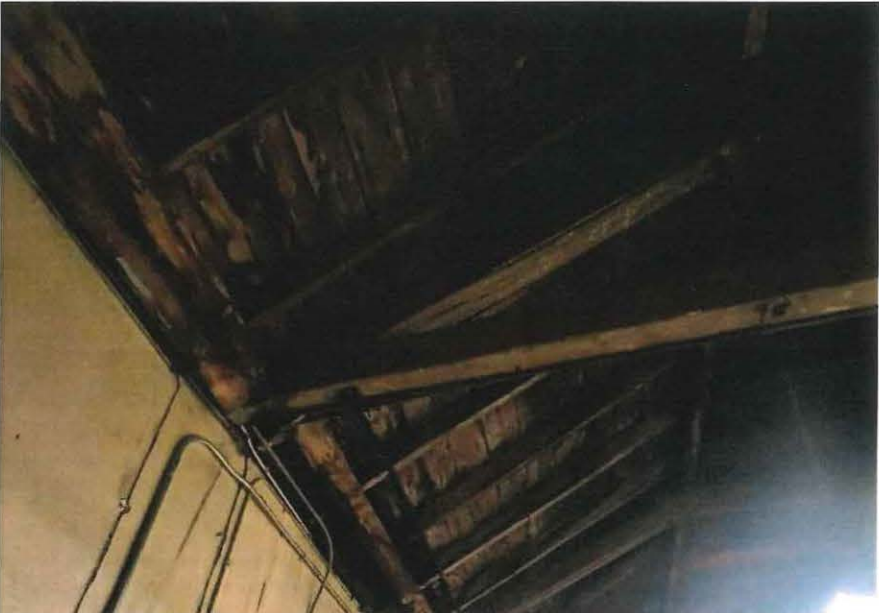
MIDDLE BUILDING EXISTING DETERIORATED ROOF STRUCTURE
