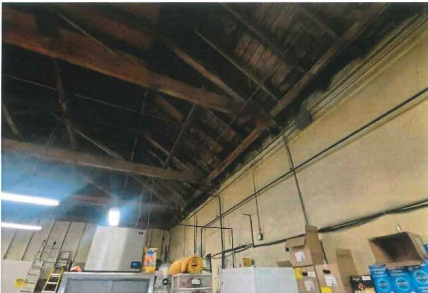
MIDDLE BUILDING EXISTING DETERIORATED ROOF STRUCTURE
