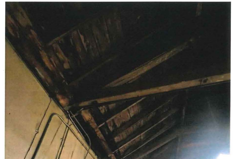
MIDDLE BUILDING EXISTING DETERIORATED ROOF STRUCTURE
