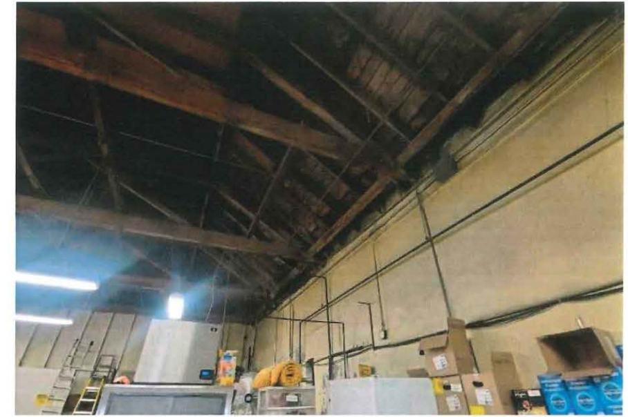
MIDDLE BUILDING EXISTING DETERIORATED ROOF STRUCTURE
