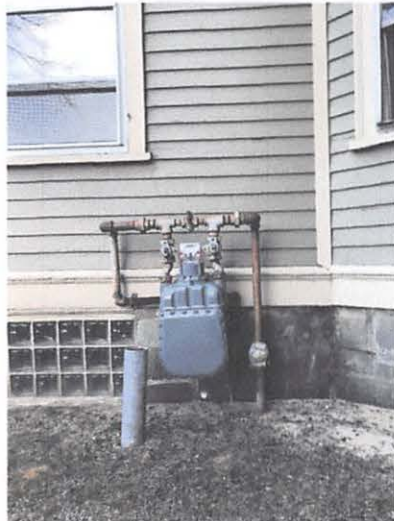
Just One Gas Meter for the Property
