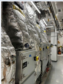
Suite 15A – Factor Bio HVAC / mechanical room
