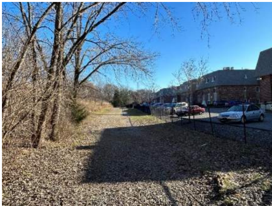
Photograph #19 Southwestern slope facing Briston Arms Apartments. Larger trees growing from slope along vent trench.
