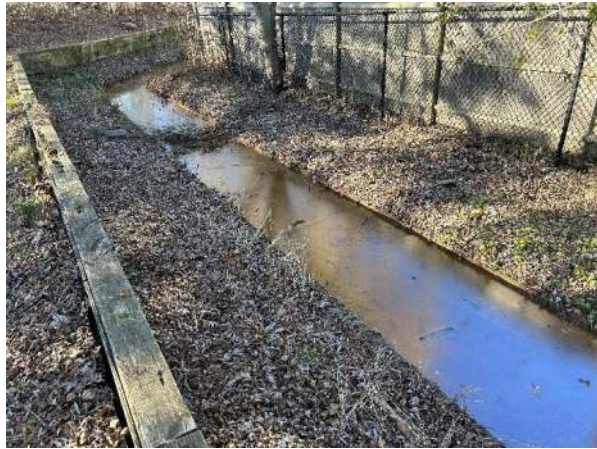
Photograph #42 Iron Flock in drainage channel between vent trench and Bellis Circle.
