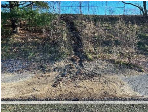
Photograph #43 Desire path turned into erosion washout on Northeast slope between soccer fields 1 and 2.
