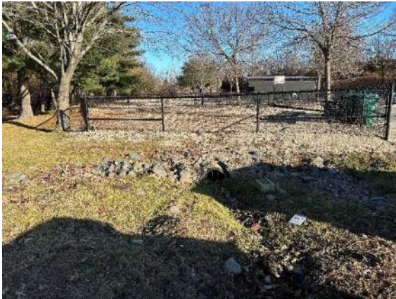
Photograph #39 Rip rap swale with drain next to dog park.
