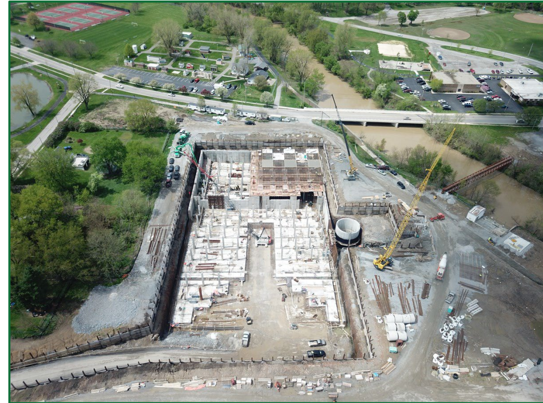
13,000,000 gallons CSO Tank Lima, Ohio
