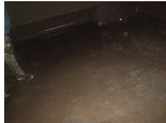
P3 Storage tank after removal of sediments. Upstream side of flush gate at upper left
