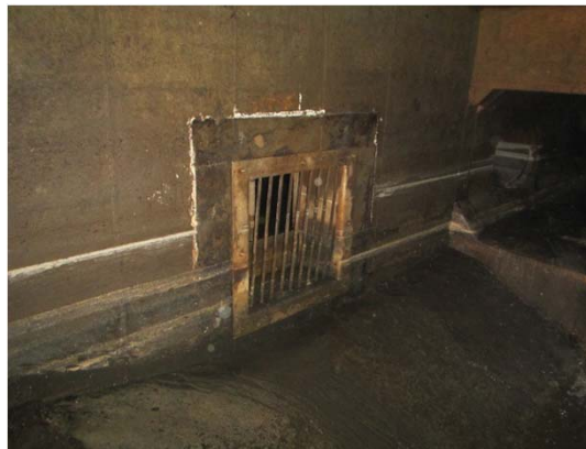
P5 Bar rack leading to pump chamber after removal of 15" PVC pipe and wooden cover
