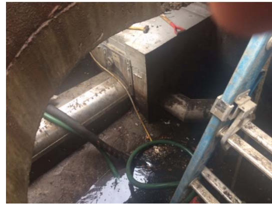
P13 Looking downstream at elevated weir with bending weir (left) and vortex throttle (right)
