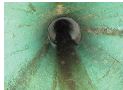
P15 Looking upstream into newly installed 24" PVC pipe inserted into existing bell
