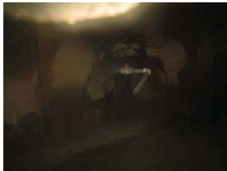
P8 Looking upstream within 4'x10' drain at bulkhead & air vent in 24" RCP dry weather lateral connection
