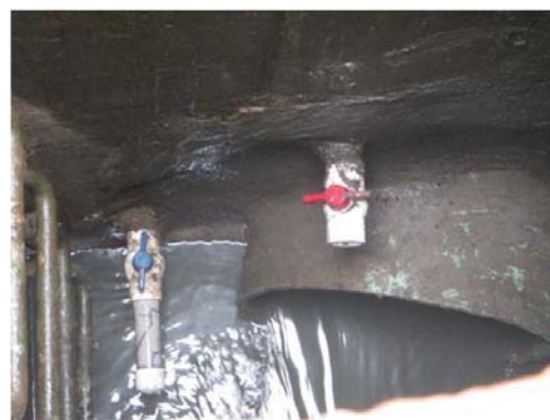
P11 Looking upstream at bulkhead with air Vents in MWRA's 48" sewer on Wheeler St.
