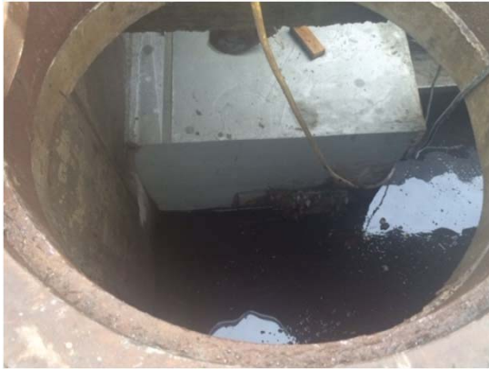
P12 Looking upstream at elevated weir with flap gate at outlet of vortex throttle
