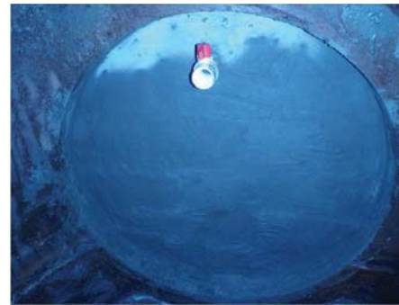
P9 Looking downstream at bulkhead with air vent at end of MWRA's sewer in rotary
