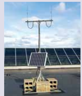
Rooftop receiving unit for daily readings from customers' meters.
