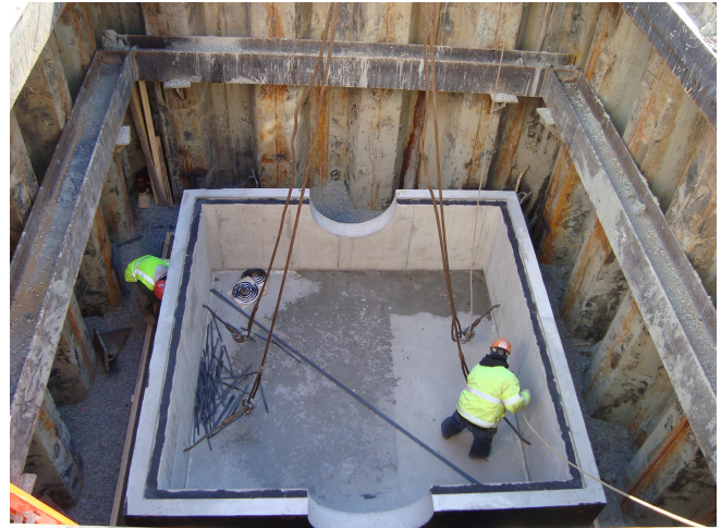
Stormwater tank under Hovey Avenue
