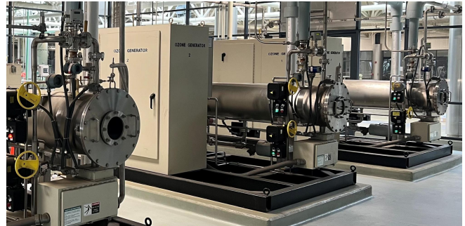
Ozone generators at Cambridge water treatment facility.
