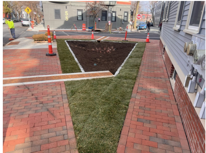
Bio basin constructed on Webster Avenue
