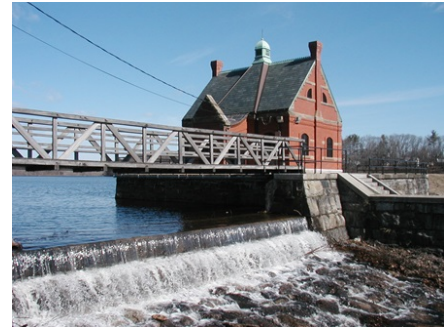
High flows passing through the auxiliary spillway of the Stony Brook Dam after a hurricane
