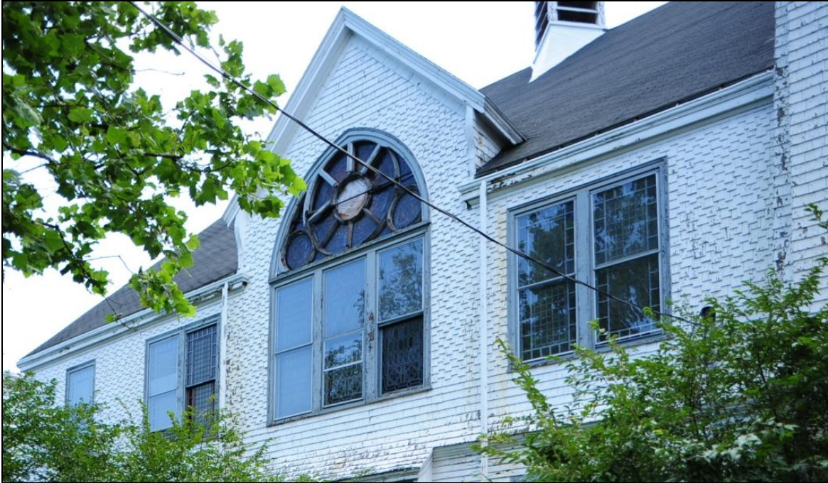
Fig. 5 Perry Street elevation, 2 nd floor, showing deteriorated wood framing of stained glass window. CHC photo, 2012.
