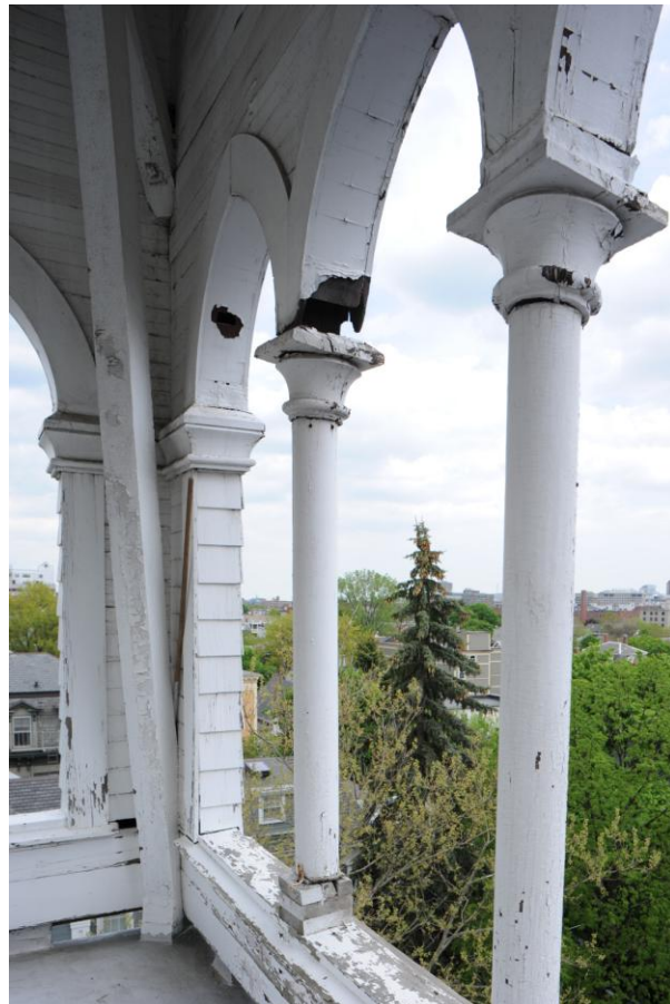
Fig. 10, Interior of belfry, showing wood deterioration. CHC photo, 2009.
