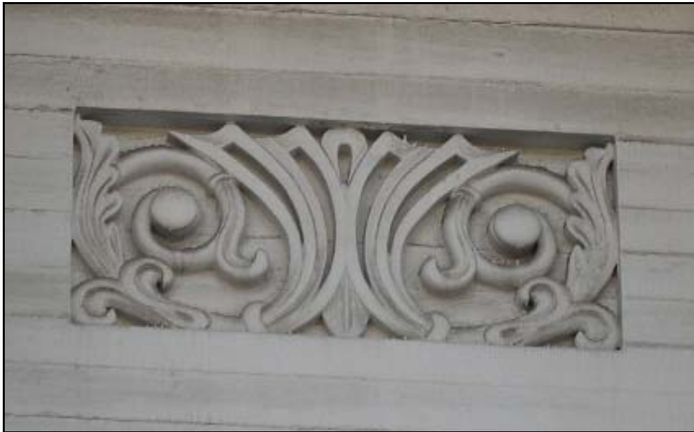
4. 1803 Massachusetts Avenue, March 2009. Showing carved detail above front entrance doors. Photo by Sarah L. Burks.
