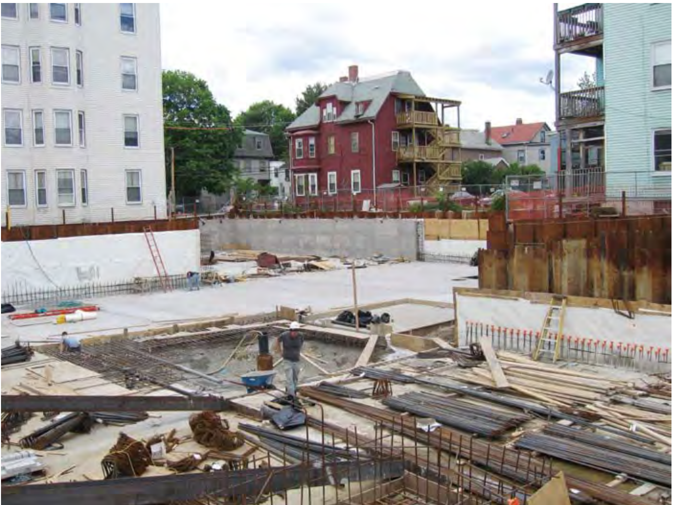
Mixed-income housing being built on the site of a former nightclub near Central Square.
