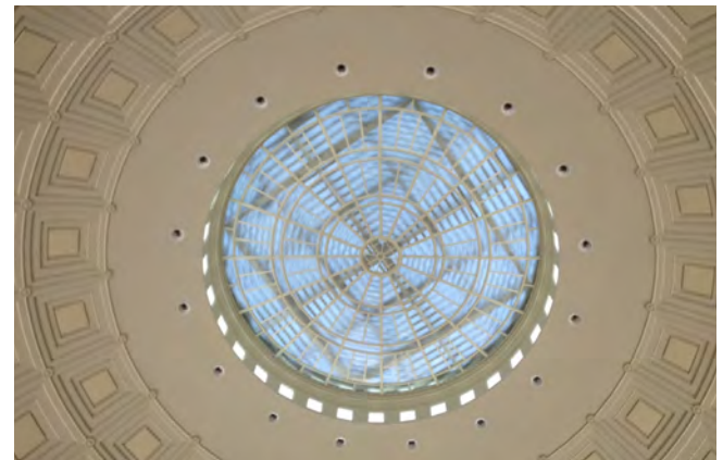
Newly renovated oculus atop the Great Dome, as seen from Barker Library
