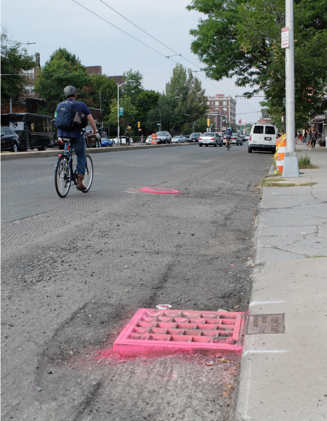
Street repaving zone featuring manholes painted with reflective pink paint.
