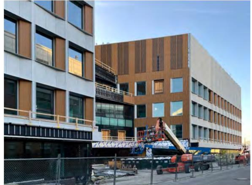
Forecourts, open to the street, can create welcome interruptions in the streetwalls of long buildings.
