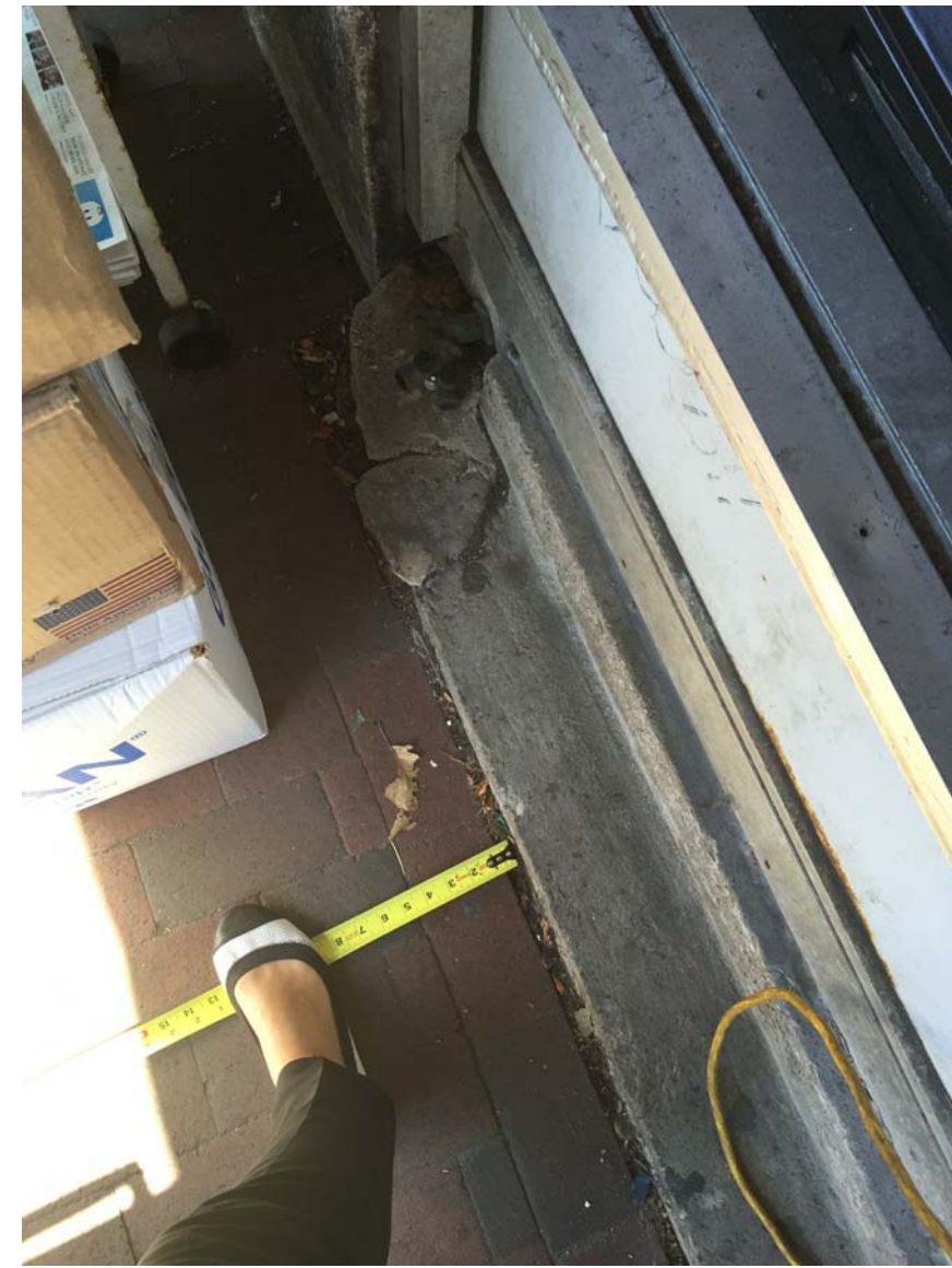
CLOSE UP OF BRICK AND CURB CONDITIONS
