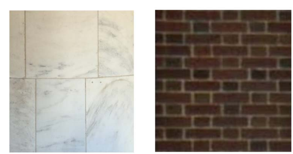
EXISTING MARBLE TO REMAIN AS IS EXISTING BRICK TO REMAIN AS IS
