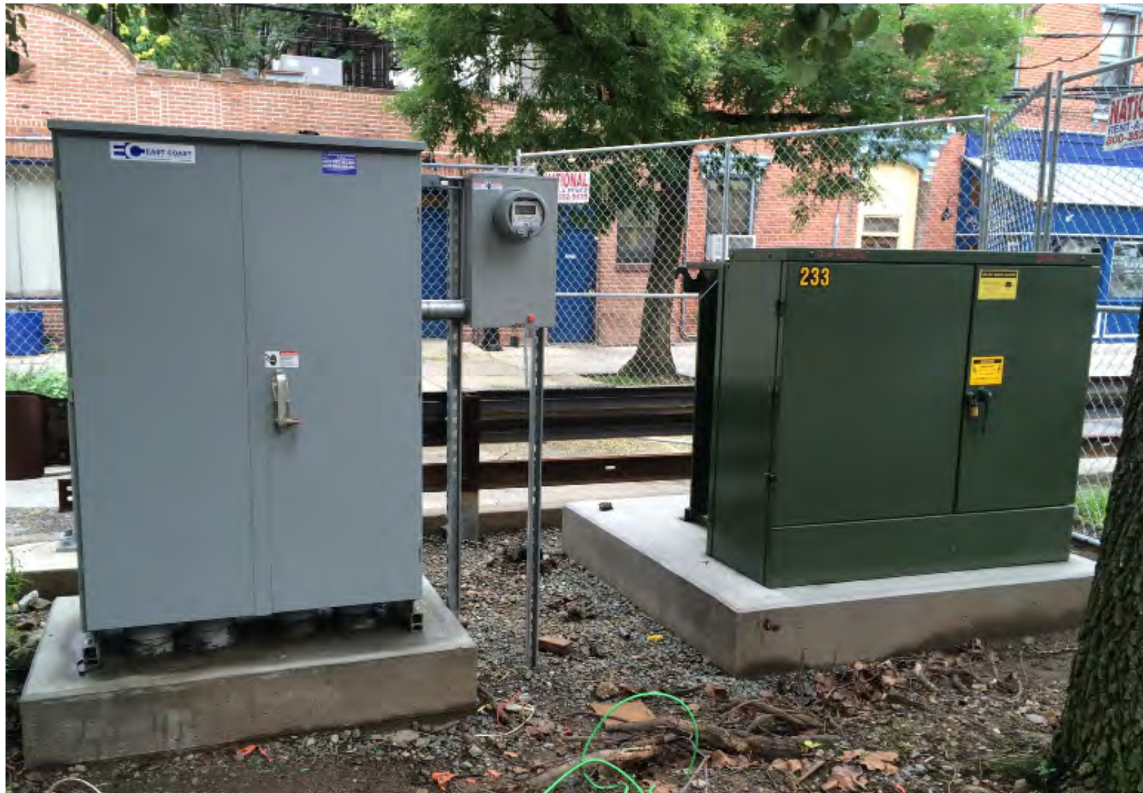
Transformer & Metering Cabinet
