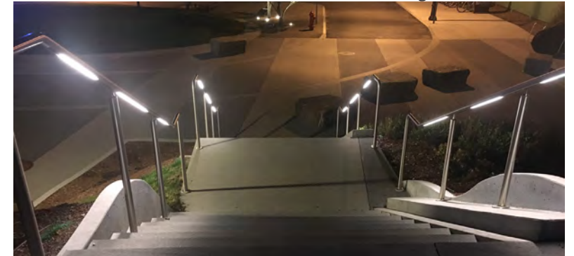
3 Existing Murphy Staircase Handrail Lighting Fixtures
