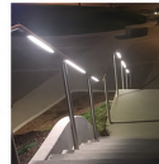
3 Existing Murphy Staircase Handrail Lighting Fixtures
