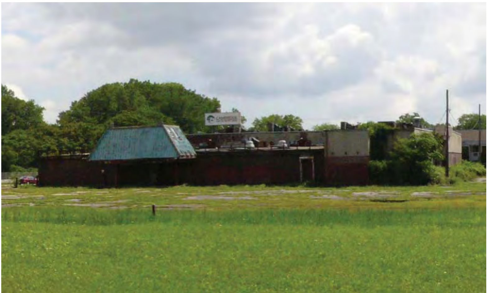
Existing dilapidated building
