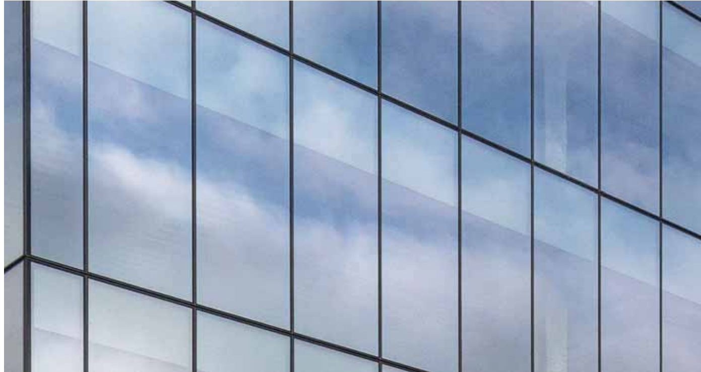
CURTAIN WALL SYSTEM WITH VISION AND SHADOW BOX GLAZING (PIER 4 OFFICE BUILDING)
