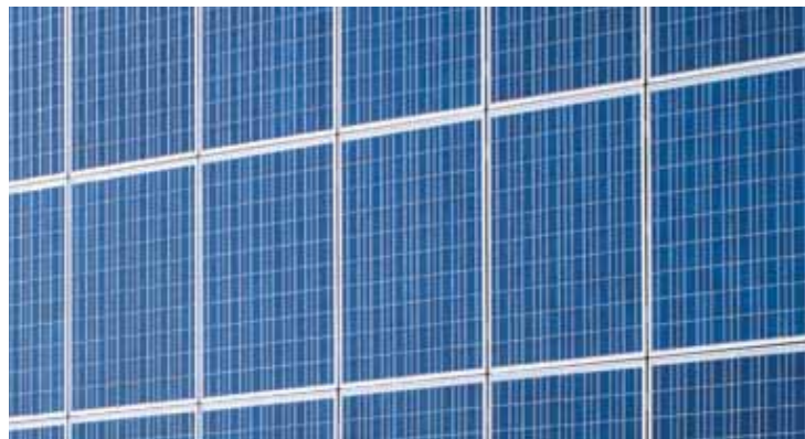
PHOTOVOLTAIC PANELS AT MECHANICAL PENTHOUSE (ANIMO LEADERSHIP CHARTER HIGH SCHOOL)
