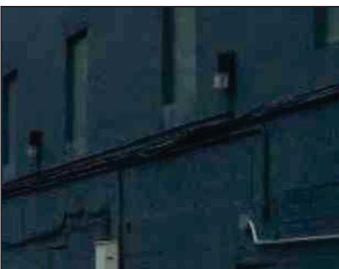
TYPICAL REAR BUILDING WALL LIGHTS
