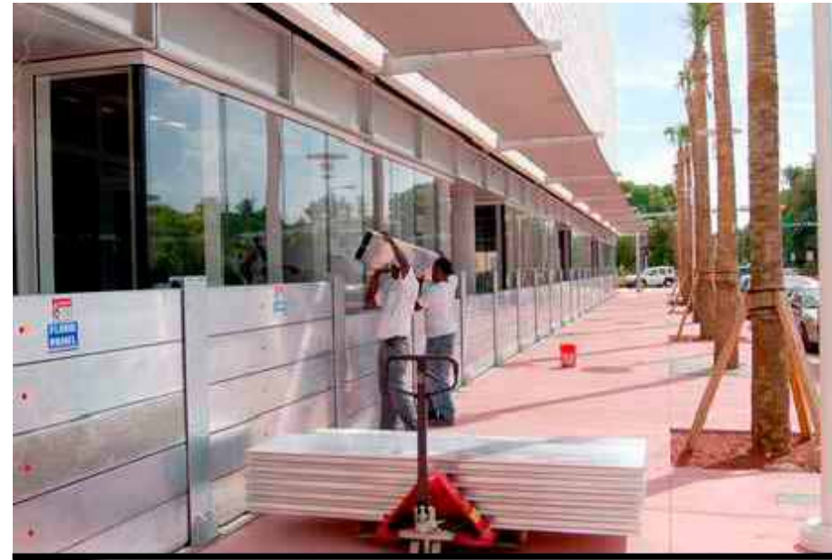
B: Flood Log
