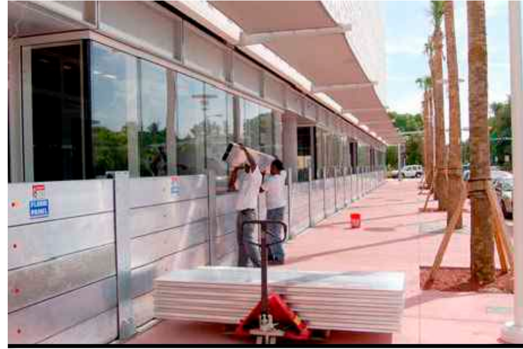
B: Flood Log
