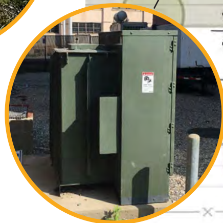
Retained Utility Cabinets
