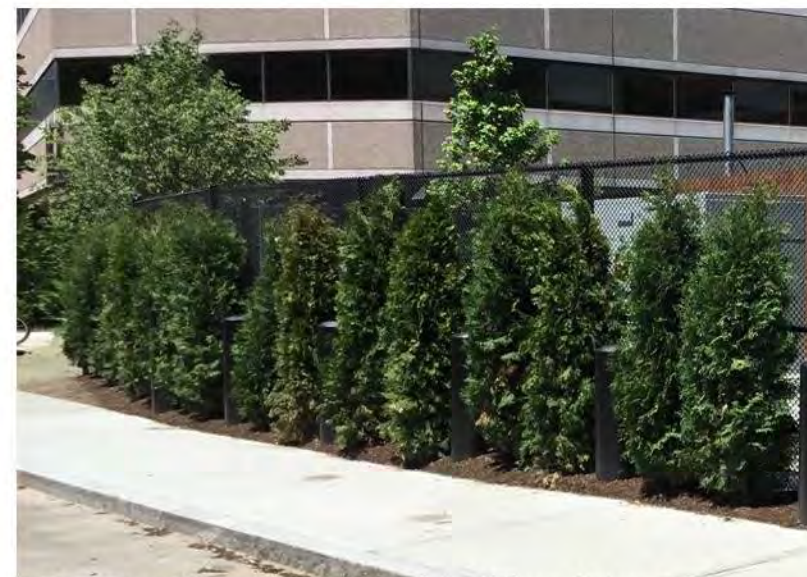
Evergreen Screening at Electrical Transformers
