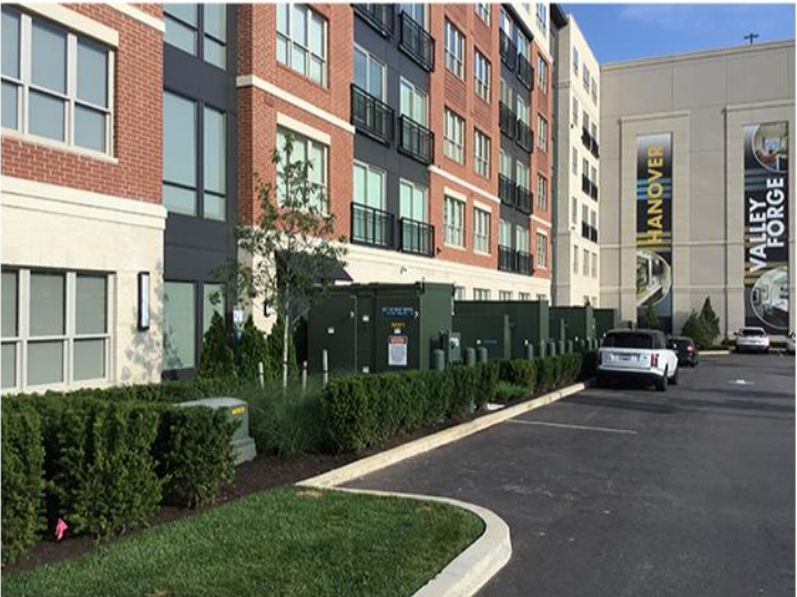
Typical Transformer Screening
