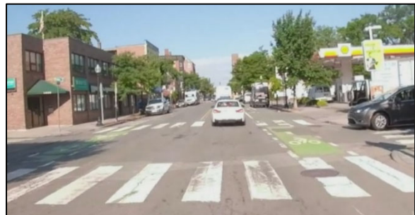
Image 4: Faded pavement markings can be observed, especially green bicycle pavement markings.
