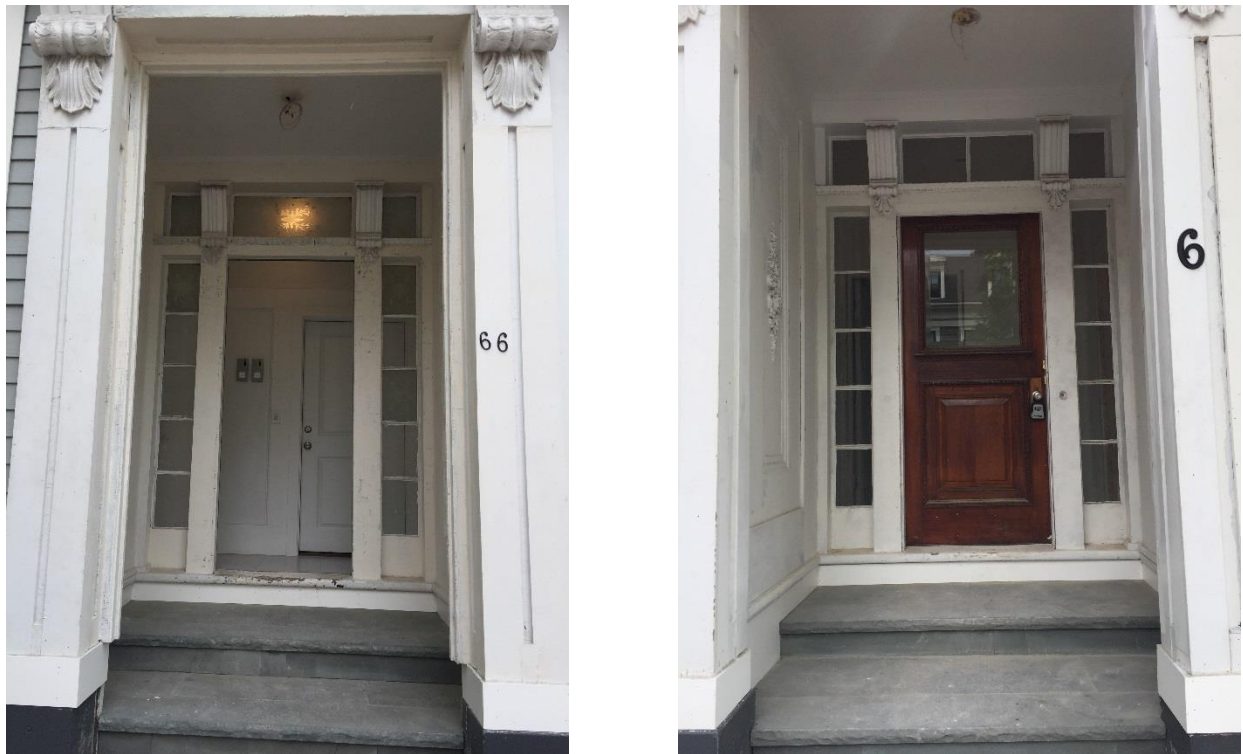
Recessed entries at 66 (left) and 68 (right) June 2017. The trim and etched glass, where existing, has been preserved in place, but a replacement door has not yet been installed at 66. Finish carpentry and paint are incomplete.
