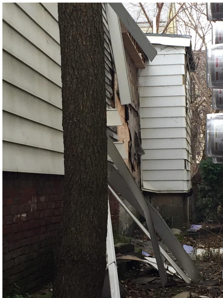
9 Pine St., north side of the ell (beyond tree trunk) and rear addition, 2019
