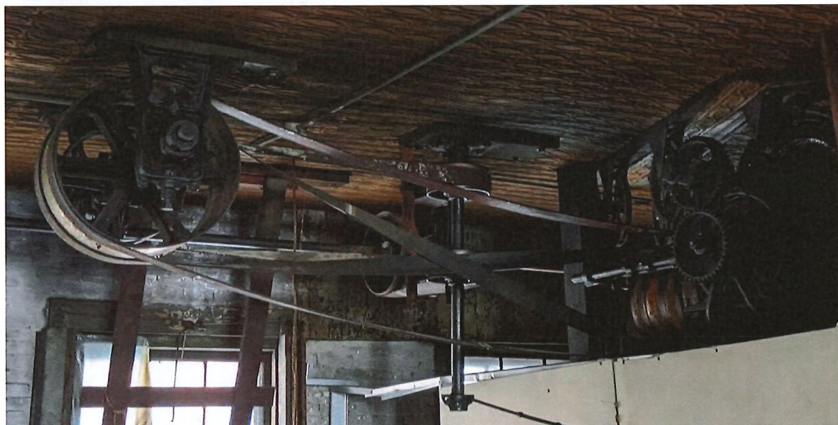
Line shaft, first floor (top); elevator mechanism, second floor.
