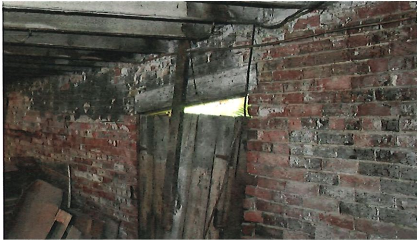
Figure 6 Lintel which is no longer horizontal
