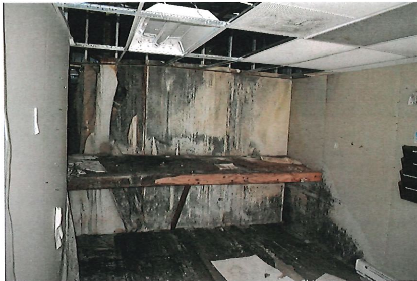
Figure 15 Water damage and mold on interior finishes
