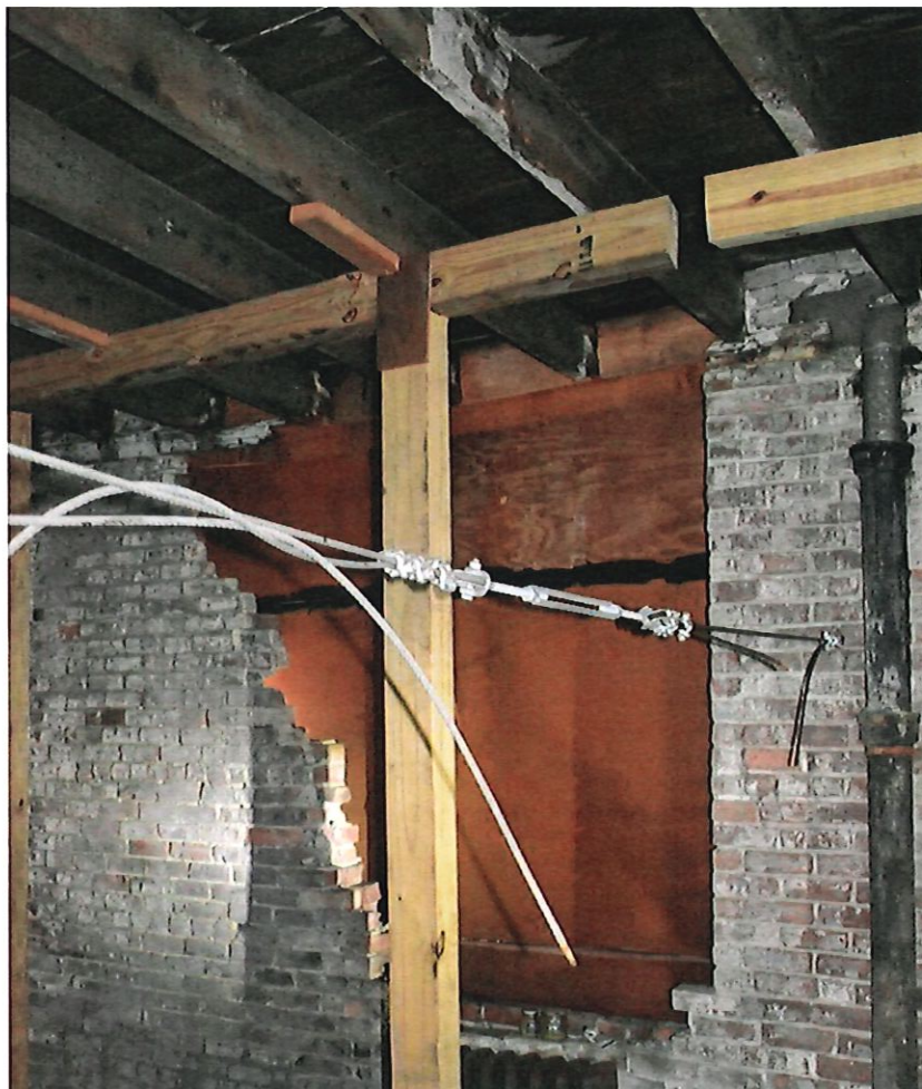
Figure 7 Area of collapsed brick wall and shoring of roof joists
