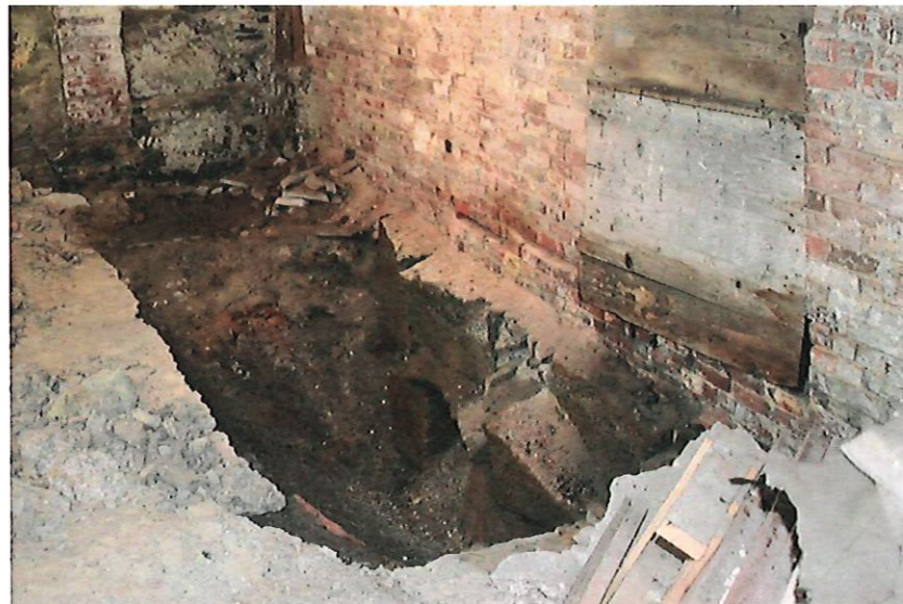
Figure 5 Bulging at base of perimeter bearing wall
