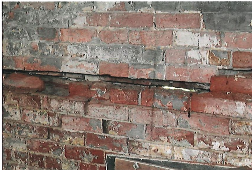
Figure 3 Horizontal gap in perimeter bearing wall
