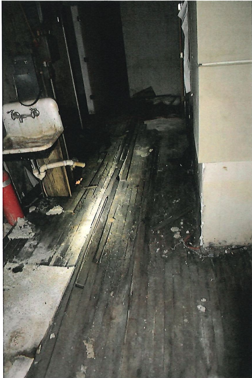
Figure 11 Uneven walking surface on first floor
