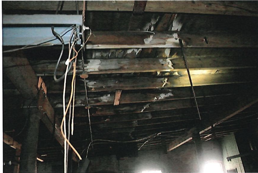
Figure 13 Water damage on roof joists
