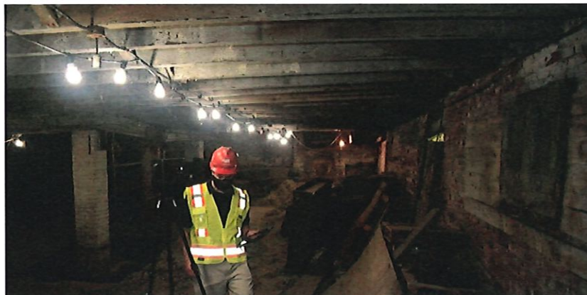
Figure 9 Joists supporting first floor, noting varying amounts of inclination off horizontal
