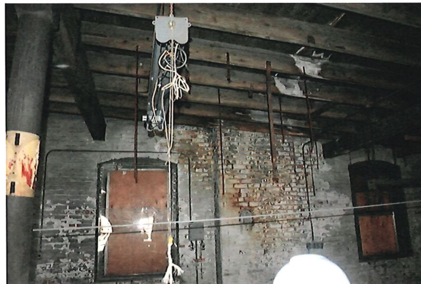
Figure 14 Water damage on roof joists and exterior walls
