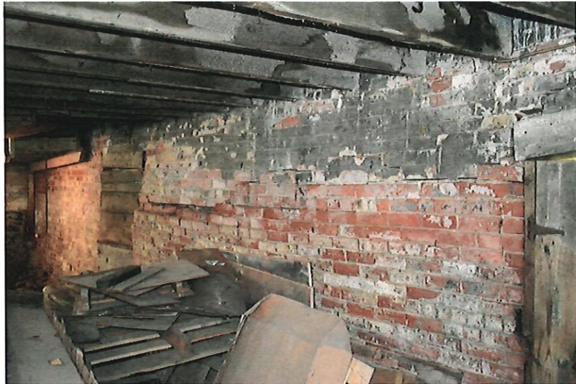
Figure 4 Step cracking along the length of the basement wall
