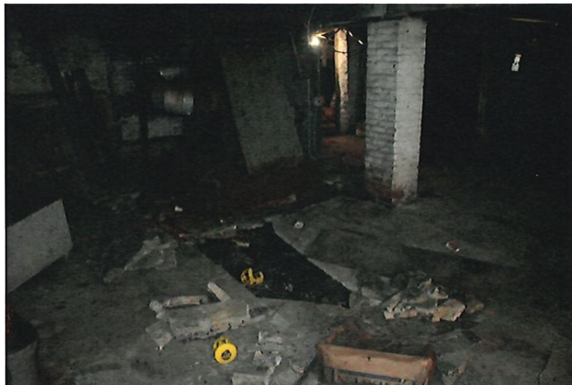
Figure 1 Damaged slab on grade in basement
