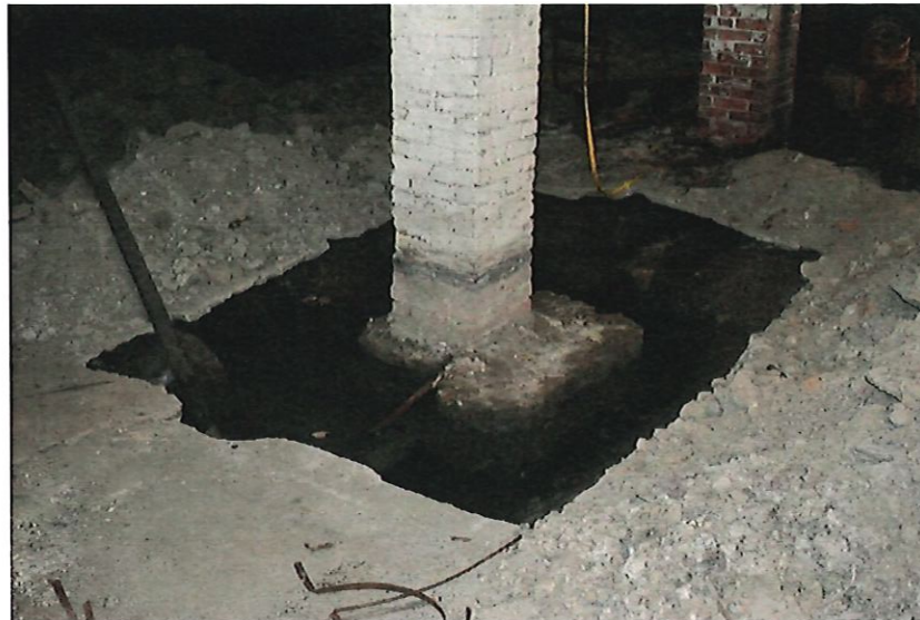
Figure 2 Exposed spread footing under brick pier in basement
