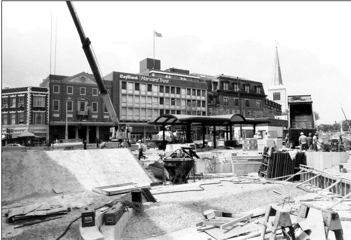
Harvard Square plaza under construction in Summer 1985. The Pit is in the foreground. Photo by Jane Erwin. Community Development Department Collection, CHC Archives.
